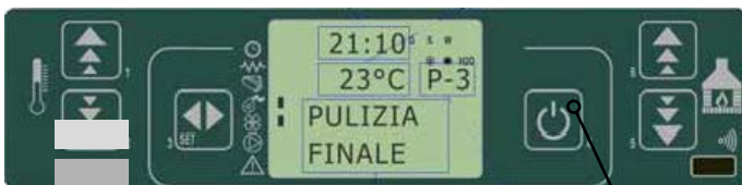
fig. 32 control panel - final cleaning
