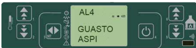
fig. 43 control panel - flue gas extraction fan alarm
