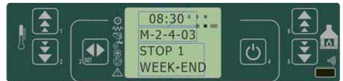
fig. 23 control panel - weekend programming
