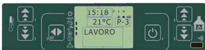
fig. 25 control panel - operating condition
