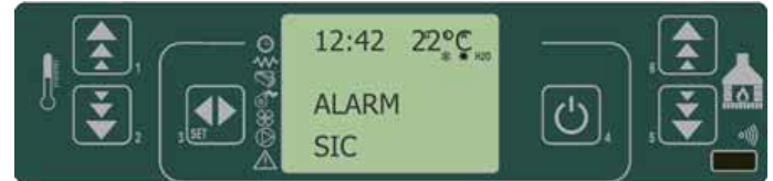
fig. 38 control panel - general thermostat alarm
