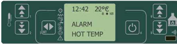
fig. 34 control panel - flue gas overtemperature alarm
