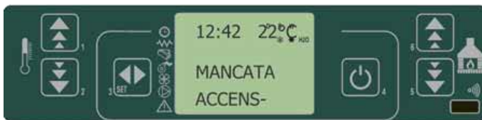
fig. 35 control panel - failed ignition alarm
